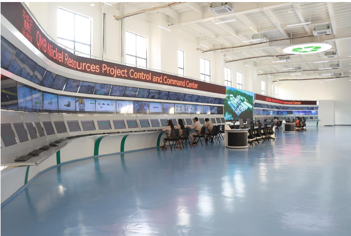
Figure 2: Central control and command centre of QMB's HPAL nickel project
