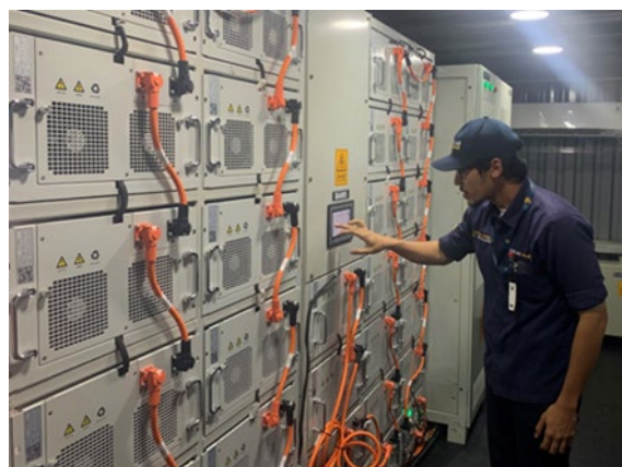
450kWp solar system fully commissioned
