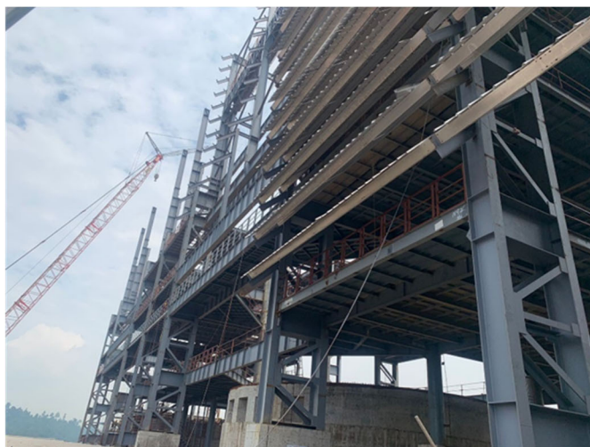
Base of ONI Electric Furnace
