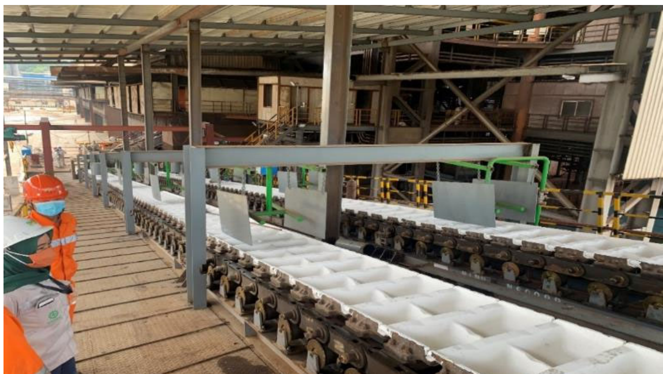
Commissioning of ingot conveyer at Ranger Nickel
