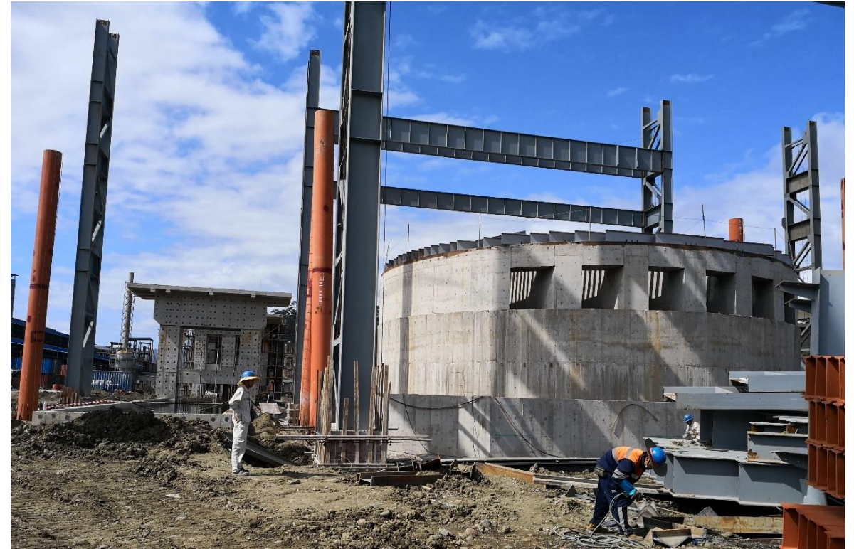
Base of Electric Furnace
