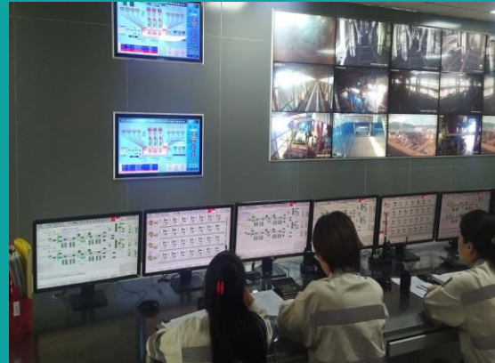
RKEF Control Room
