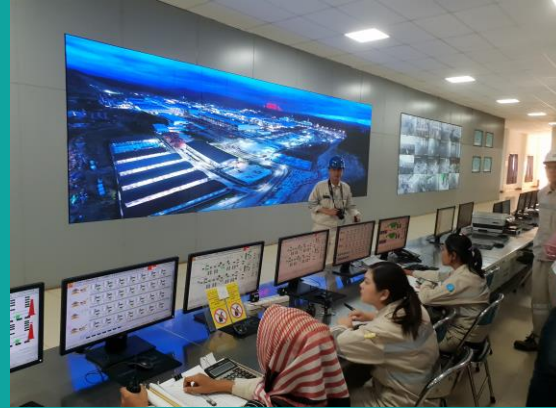
RKEF Control Room
