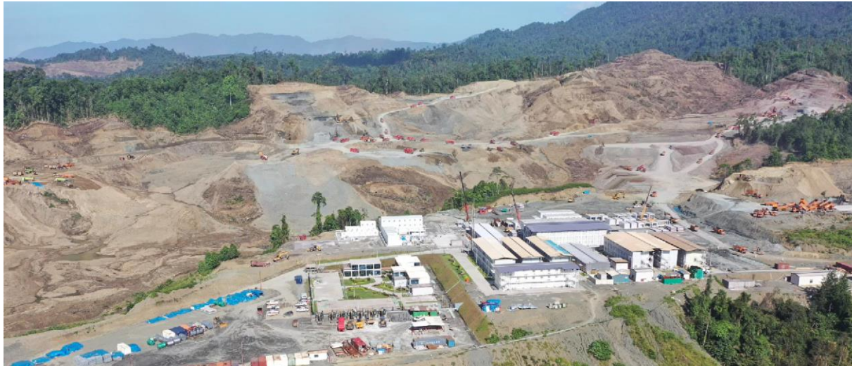
Earthworks and footings at ENC largely complete in readiness of concrete pouring and plant erection
